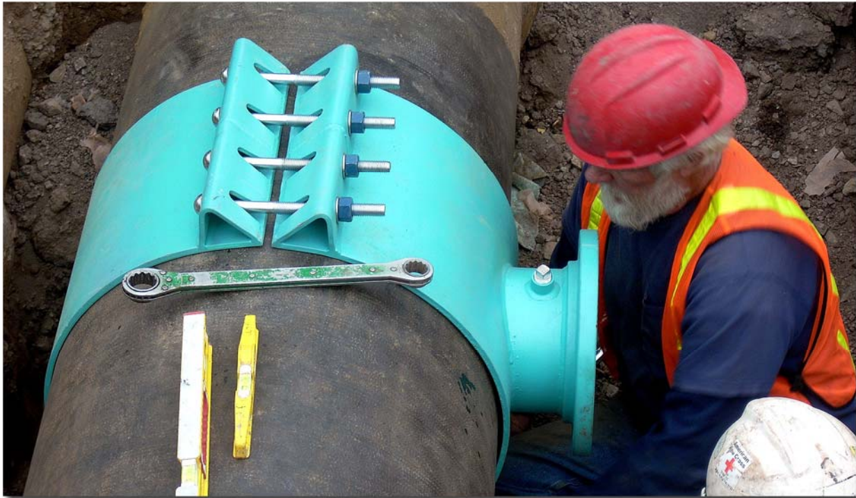
8-INCH WET TAP ON EXISTING 24-INCH RAW WATER LINE (at Lift Station)
