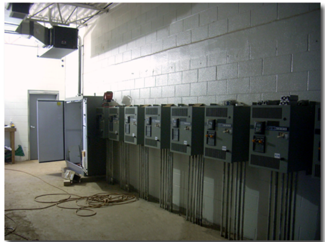
Operations PLC & VFDs for RAS & WAS Pumps
