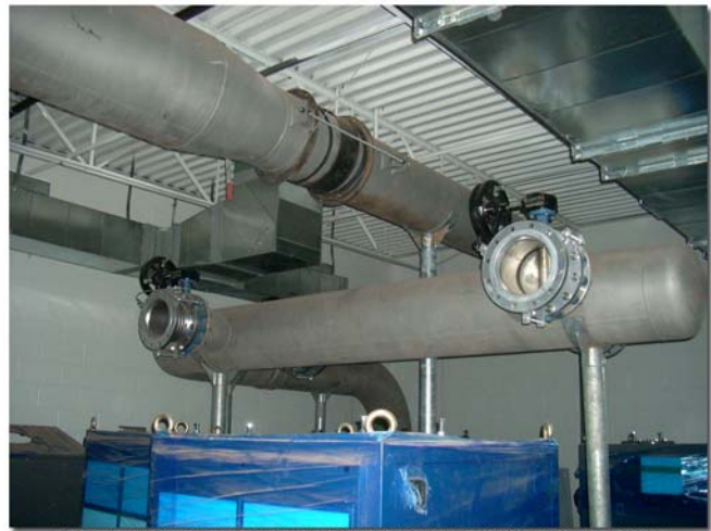
STAINLESS STEEL AIR DISTRIBUTION PIPING MANIFOLDS - BLOWER ROOM
