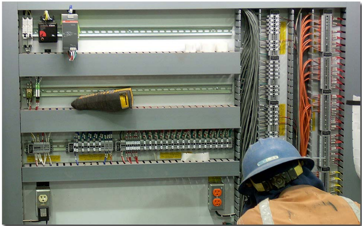
Looking Inside the BioSolids PLC
