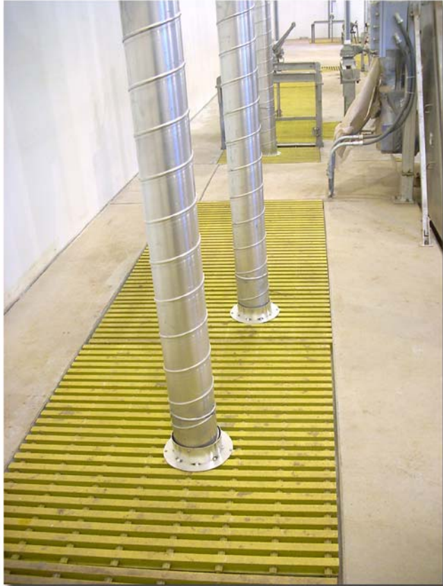
Influent Bypass Channel-Odor Control Ducts
