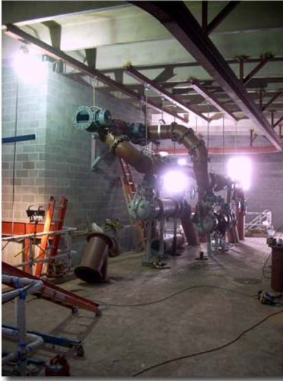
Lift Station-FM Discharge Pipe
