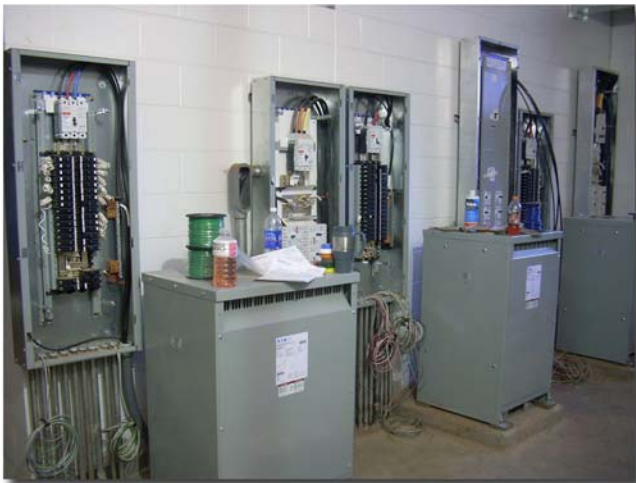
Operations - Power Panels & Transformers
