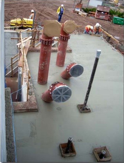
LIFT STATION - PIPE OPERATIONS ROOM
