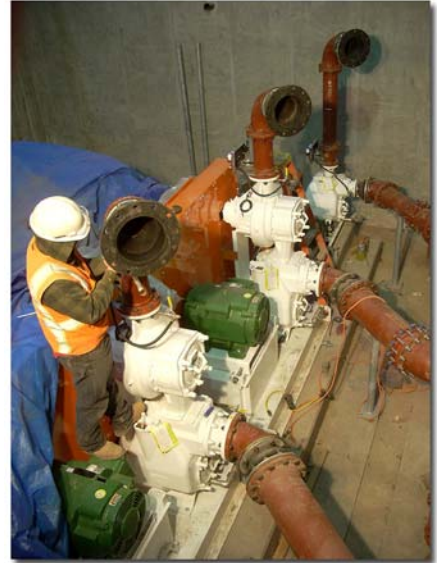
LIFT STATION-NORTH PUMP ROOM
