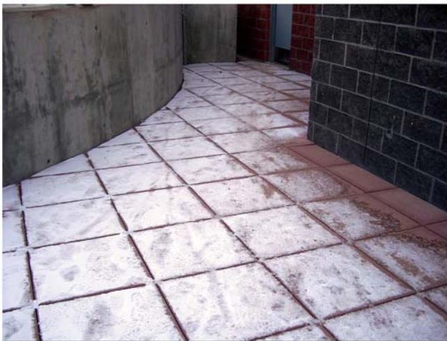
PAVER TILES BETWEEN OPERATIONS AND CLARIFIERS
