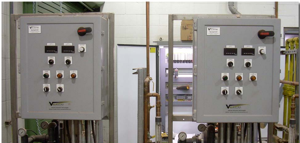
Local Control Panels for the Polymer Feed System
