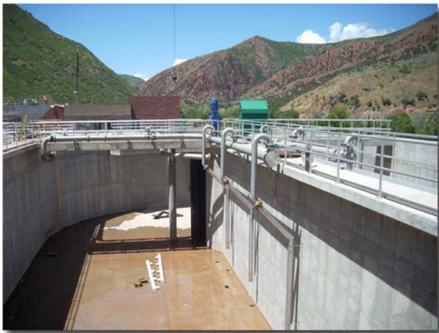
Stainless Steel Air Distribution Piping - O Ditches
